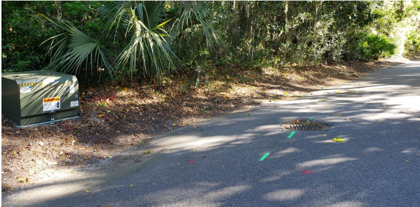
Electric for H Building – runs straight across drive from the Main green electric box
