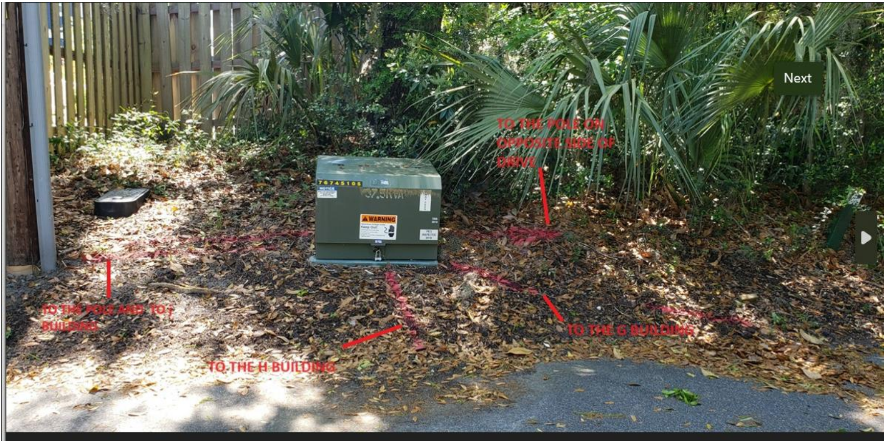
Box where all the electrical comes together – opposite side of 211 driveway from H building
